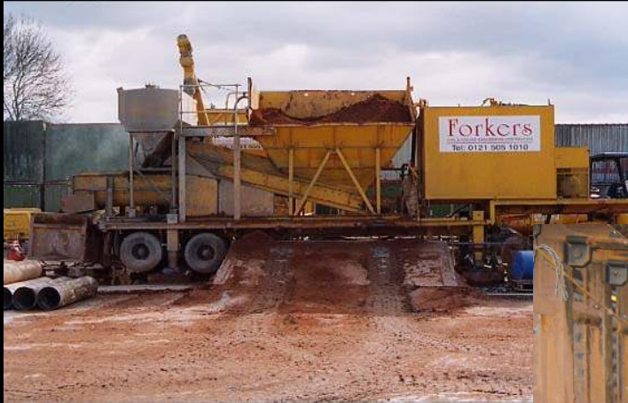
Sand mixing and pumping plant
