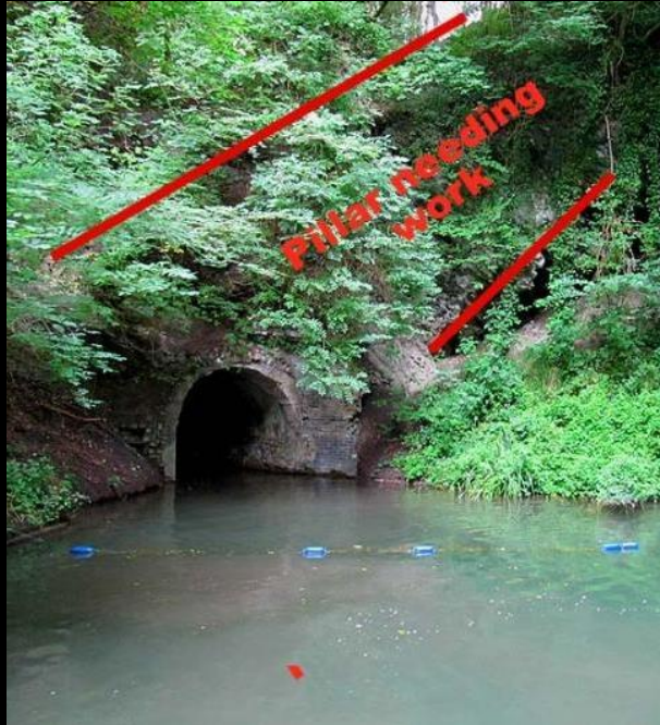
Weak Rock Pillar over tunnel entrance
